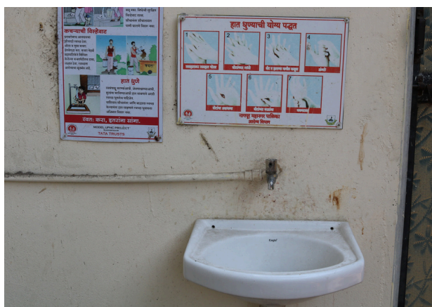
Figure 18: Indora UPHC Handwashing Point Patient Toilet
